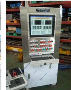
[Main Control Console]
